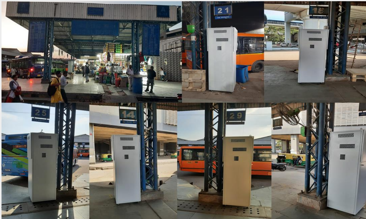
Figure 8. Picture of APS installed at the Anand Vihar ISBT
