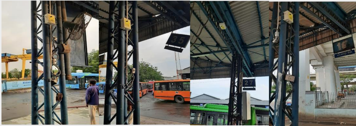
Figure 4. Picture of sensors (S1-S4) installed at the site
